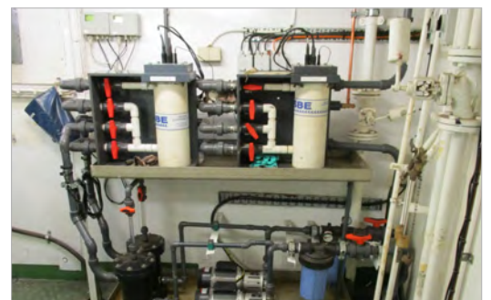
KATflow 100 installation as part of a thermosalinograph system on the research vessel METEOR.
